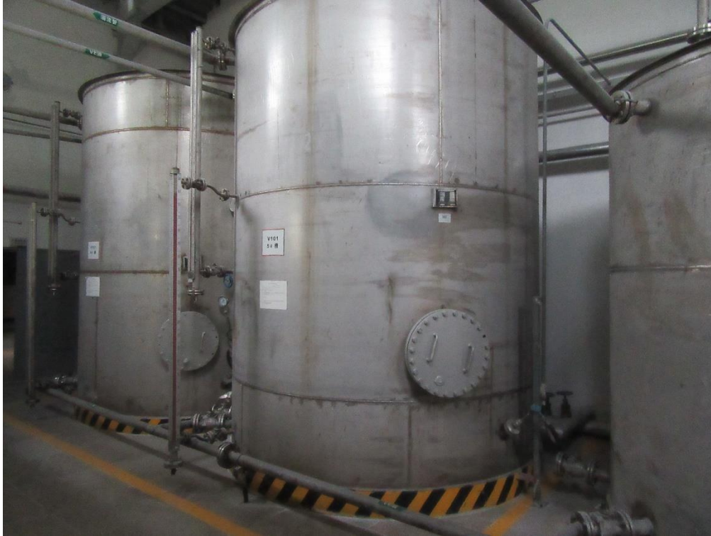
Figure A2.9. Locked, secure, and isolated raw material tanks
