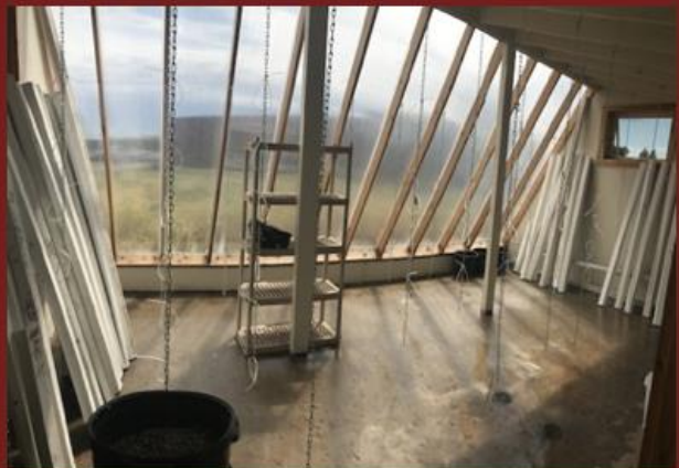
The interior of the greenhouse with hanging gutters waiting to be installed
