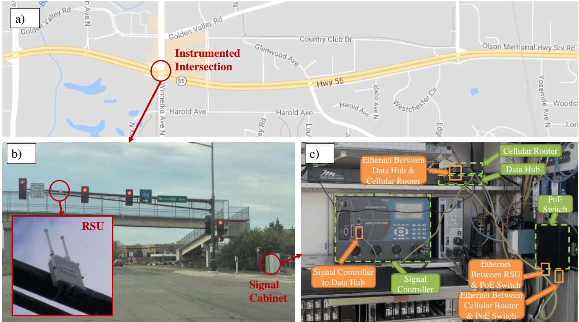
Figure 6.8 Living lab intersection instrumentation: a) location of the instrumented intersection (between Trunk Highway 55 and Winnetka Ave); b) view of the RSU mounted on the signal pole; c) inside view of the instrumented signal cabinet
