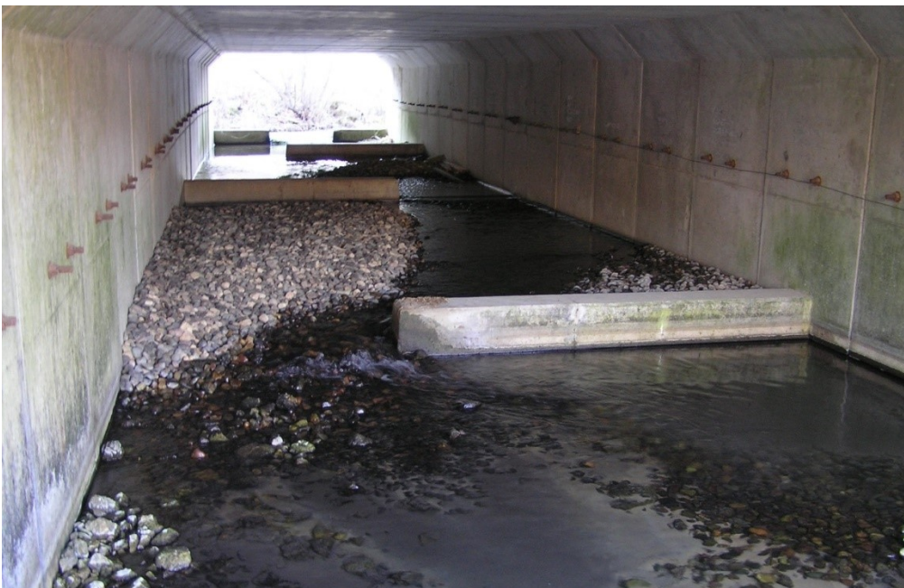
Figure 5.6.2. Alternating concrete baffles retaining gravel to cobble size material in a culvert near Red Wing, MN. Photo courtesy of B. Hansen.
