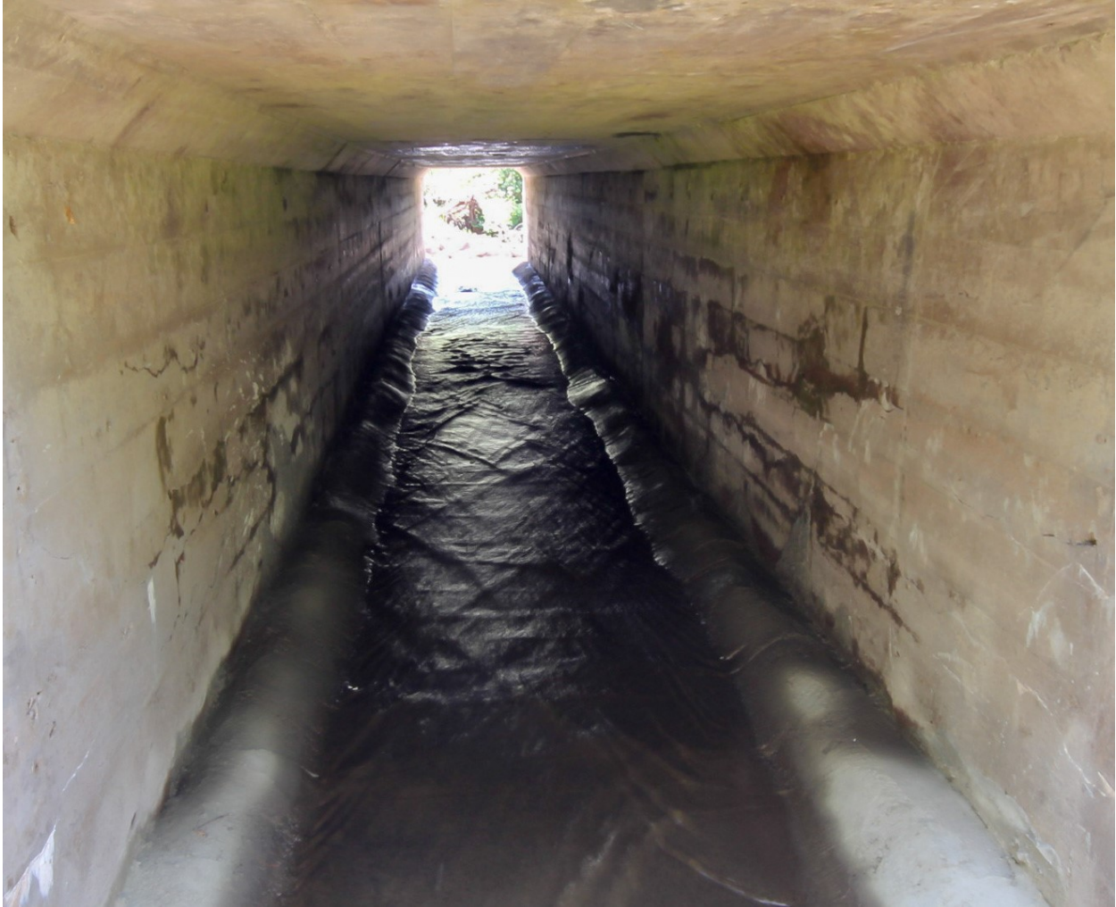
Figure 1.2.4. Excessive velocity over an extended length with no resting areas can impede fish and aquatic life movement both in culverts and adjacent channels creating a hydraulic barrier. This culvert also has shallow flow, another potential barrier to movement. Photo: Indian Camp Creek below TH61 in Cook County (P. Leete photo, 2015)
