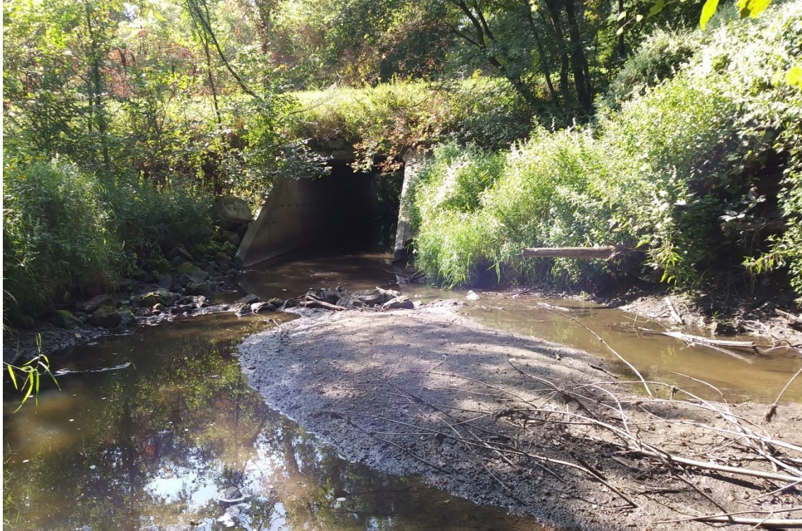
Figure 3.11.10. View of culvert inlet for Le Sueur Creek example, looking south (downstream). The east barrel on the outside of the bend conveys lower flows. The west barrel is almost hidden by vegetation growing on accumulated sediment. A mid channel bar has aggraded just upstream of a partial line of riprap.
