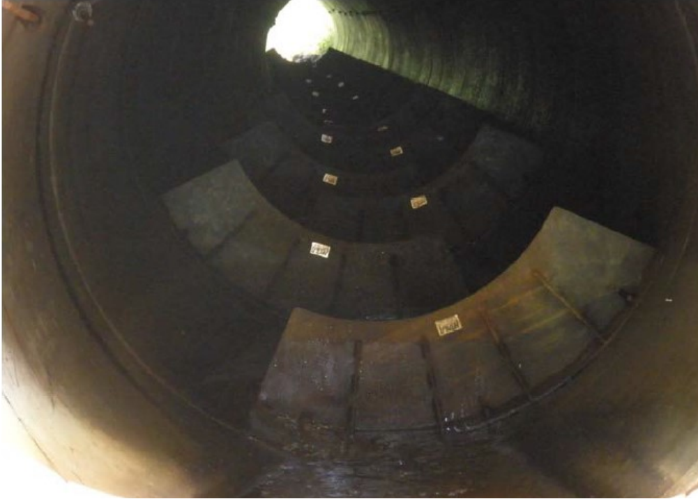
Figure 5.6.1. Steel offset baffles bolted to a round concrete culvert as a retrofit. St. Louis County (from Fig. 4.5, Hansen et al. 2009)
