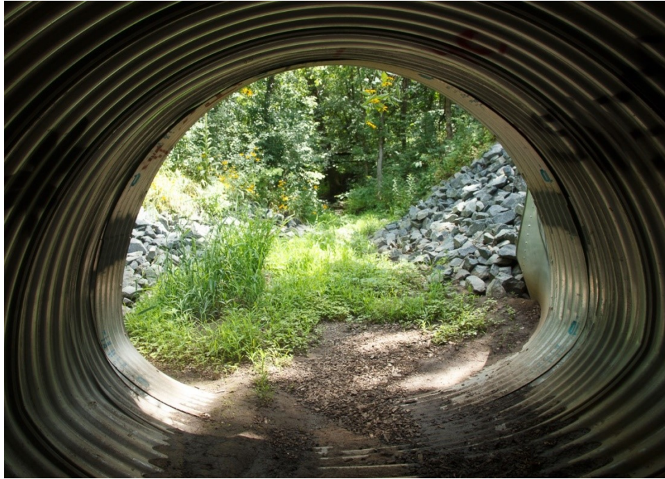
Figure 1.2.5. In this mid-July 2017 photo there is no flow through this culvert on an intermittent tributary to Lawrence Creek, a designated trout stream in Chisago County (P. Leete photo).
