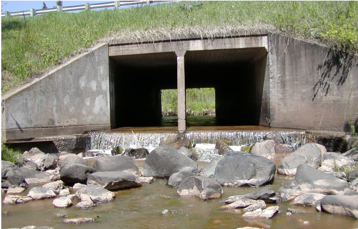
Figure 6.3.1. The significant perch and very shallow flow present several barriers to AOP at this culvert on the Nemadji River South Branch at TH 23 in Carleton County. A grade control structure was later constructed downstream (next figure). Photo courtesy of L. Aadland (2001).
