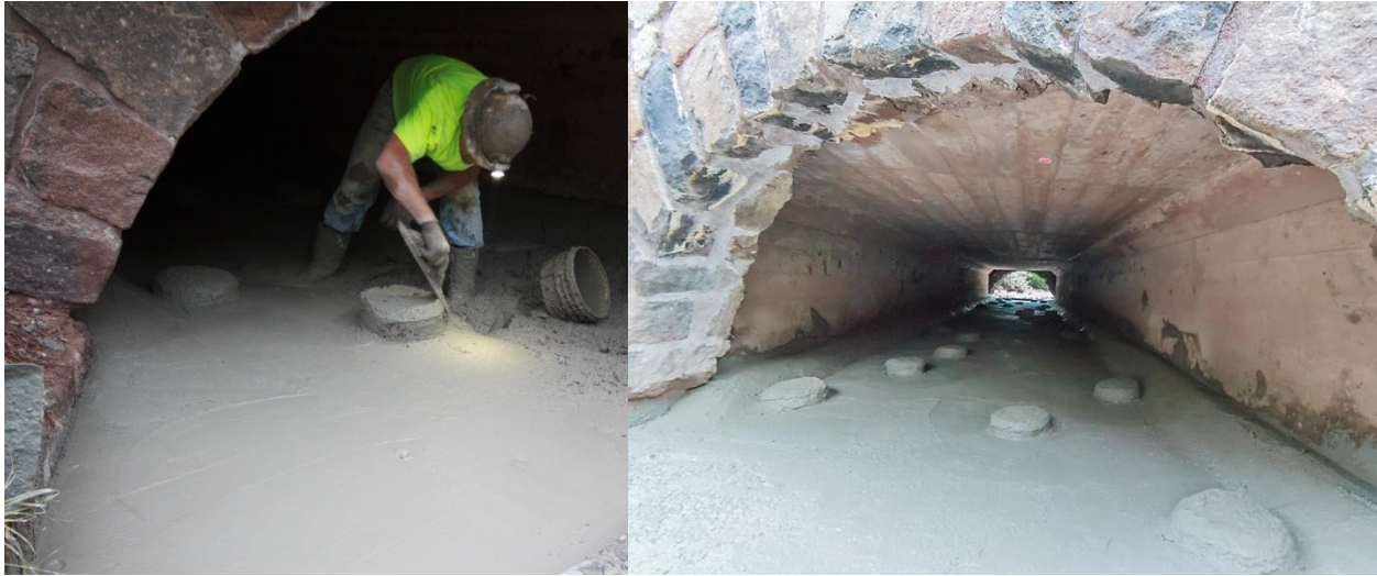
Figure 6.5.2. Paving a culvert invert prolongs the useful life but a new smooth bottom may contribute to an AOP barrier. Rock-like concrete shapes and bank lines formed monolithically with the invert pour (left) were part to this culvert retrofit to increase roughness at low flows. The culvert is on Deer Yard Creek (Spruce Creek) under TH61 in Cook County. Photos courtesy of P. Leete (2014).
