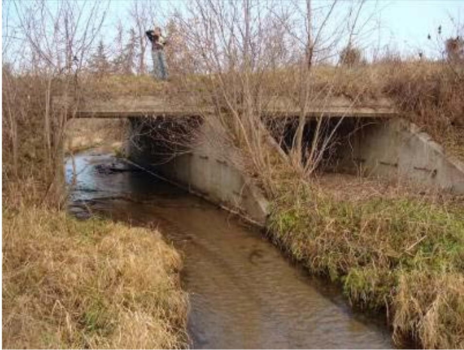
Figure 6.1.1. Low flow passes the left (channel) barrel while the right barrel is partly filled with sediment in this culvert in Goodhue County (photo from Hansen et al. 2011)
