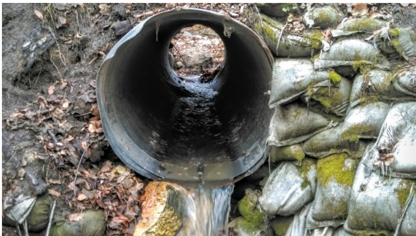
Figure 1.2.3. Perched culvert on a tributary of Seven Mile Creek, Minnesota creating a physical barrier (C. Lenhart photo)
