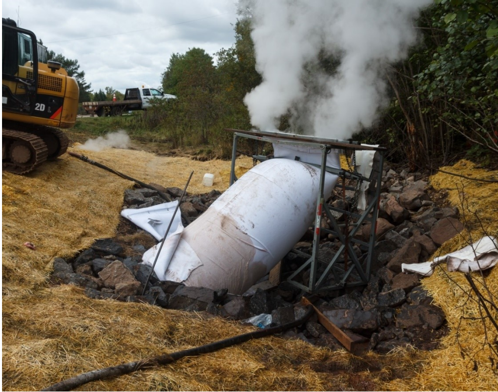
Figure 6.5.1. Cured-in place liner inserted into a culvert and inflated with steam, on TH 61 near Grand Marais, Cook County. Photo courtesy of P. Leete, 2016.
