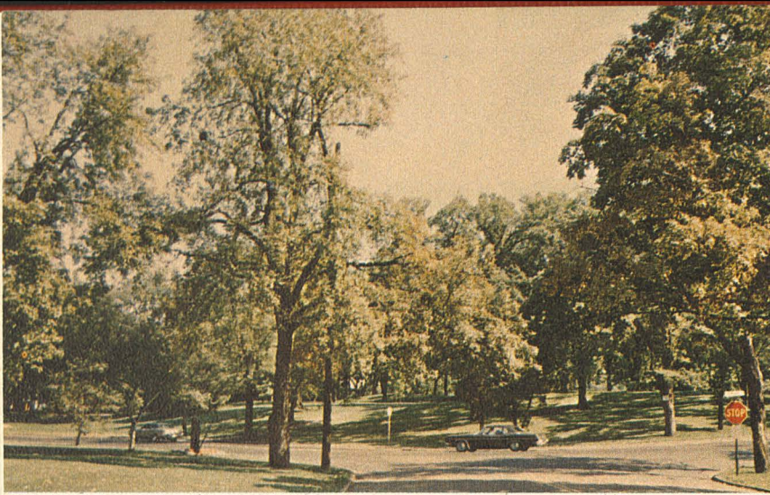
Figure 1. Soil-salt damage on trees next to heavily salted road. Brownish cast to leaves comes from marginal leaf scorch (figure 2). Tree on left has thin crown and small leaves, also characteristic of soil-salt damage.
