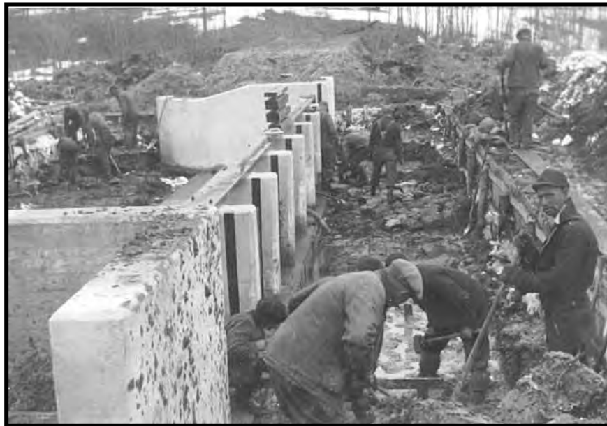
Figure 9: Construction of a Type “C” dam at Island Lake in Crow Wing County, ca. 1940. The dam has been poured, and unskilled workers appear to be laying cobbles in front of the dam in the background. Note the coffer dam on the upstream side. (Minnesota Historical Society Collections MC10.1 r6)
