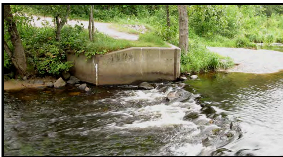
Figure 12: Modified Mayo Lake Type “C” dam, Note removal of plaque, gauge, piers and catwalk and remnant of cast concrete plaque in waterway July 2013
