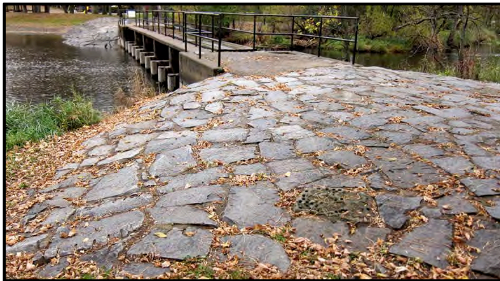
Figure 35: Dam embankment and footbridge approaches leading to the C-shaped abutments are roughly paved with salvaged granite at the Skunk River Dam in Pierz. The stonework extends down to the streambed on the upstream side providing erosion control. (October 2013)
