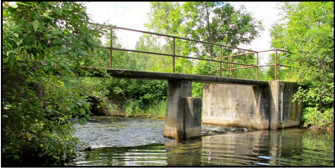
Figure 32: WPA "Type C" Ossawinimakee Dam. A good example of an intact concrete operator's platform with railings. This dam has been altered by fixing stop logs in place and sawing off the intermediary piers spaced 5 feet from the main pier and abutment. (Photo facing southwest on July 2013)
