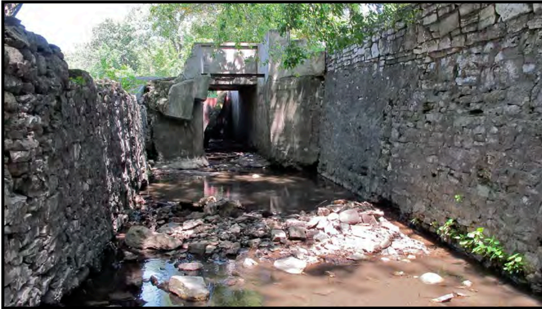
Figure 24: Lake Louise Dam at the former site of the LeRoy Mills facing north in masonry sluiceway with mill ruins to the right and sluice wall in earthen dam on the left. The upstream side of the sluice appears to have been repaired, reconfigured and narrowed circa 1925 and is closed with the replacement metal gate. August 1, 2013.
