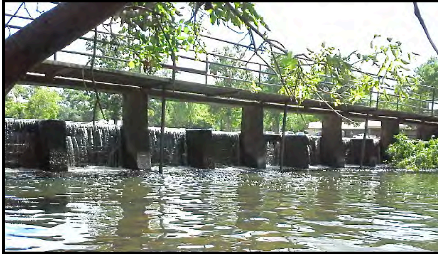
Figure 34: This view of the Skunk Creek Dam in Pierz Minnesota shows the ten-foot bays supporting the concrete operator’s platform with the intermediary piers spaced five feet apart holding stop logs. The bridge also serves as a footbridge between two sides of a WPA golf course, so there are additional supports for the pedestrian walkway.
