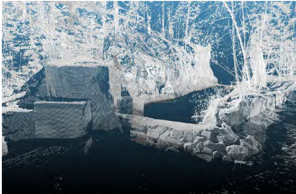
Figure 66. 3D intensity view of the Glensheen Dam, looking southwest. The water intake and filtration system is visible to the left of the dam. A 30 meter long concrete dike is partially visible to the right of the dam.
