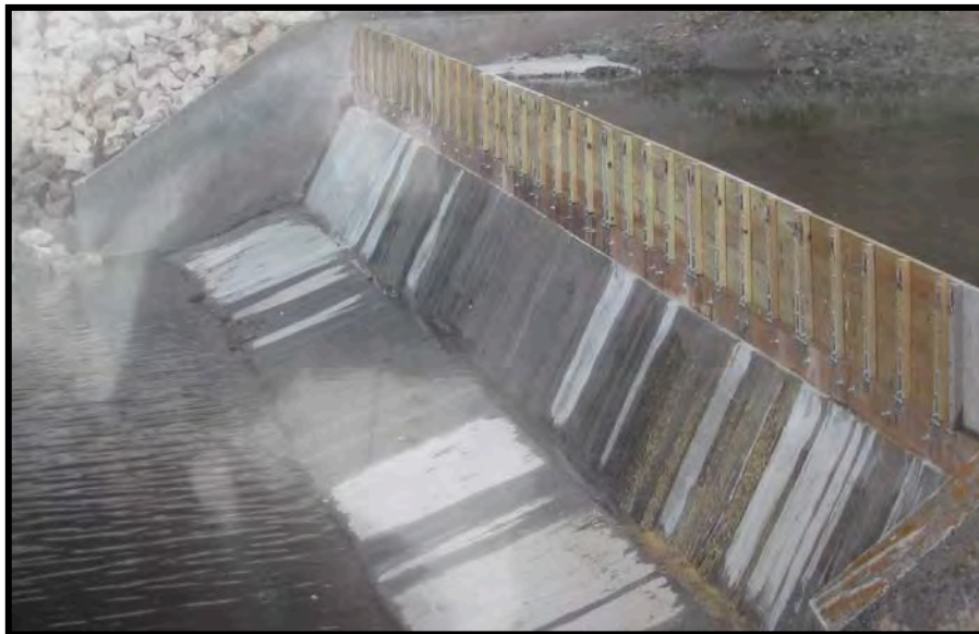
Figure 30: Schech’s Mill Dam on Beaver Creek showing flashboards on top of concrete dam in low water. Photo courtesy of Edward Krugmire.
