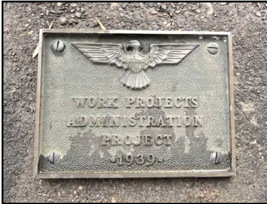
Figure 36: All WPA dams originally had a dated WPA plaque. Most also have a surveyor's benchmark and may also credit the state level sponsor. Dams originally also had water level gauges.
