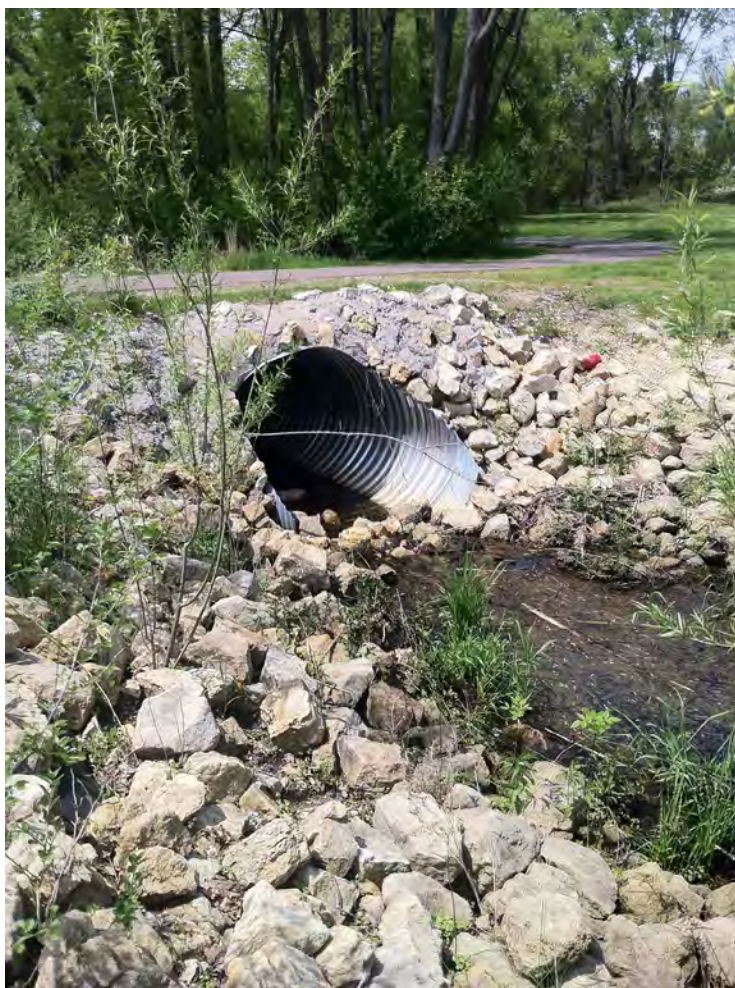
Stormwater from the Casey Lake neighborhood flowing directly into Casey Lake. Photo taken by capstone students.
