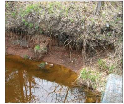
Figure 26: Side slope erosion (sloughing)
