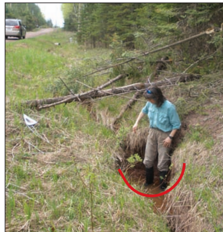
Figure 36: Example of a ditch you don't want to dig- a U-shaped ditch with vertical sides
