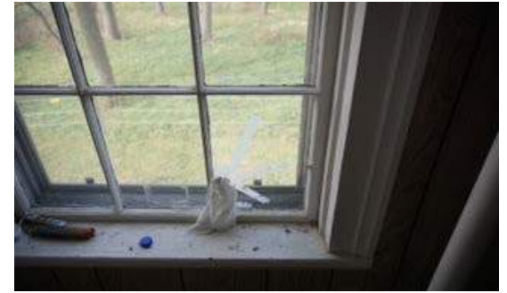
Figure 9. Window #8, lite (12) is damaged.
