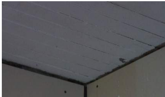
Room 5- Gaps Between Wall and Ceiling
