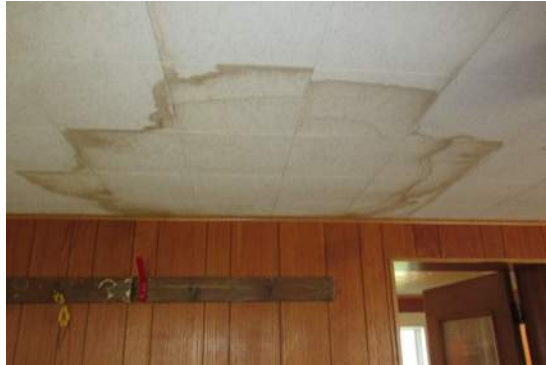
Room 4 Water Damage on Ceiling
