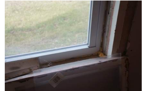
Window 5a- Close-up of Improper Spray Fill
