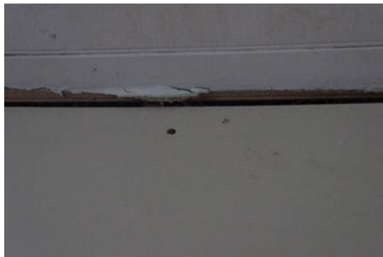
Room 5- Flaking Paint at Ceiling/Wall Edges
