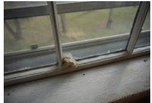
Figure 4. Window #3, lite (11) is damaged.
