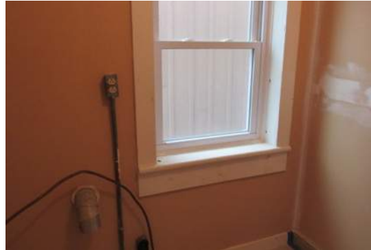
Room 1- Laundry Room Connections
