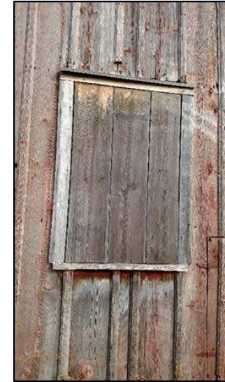
Fig. 11: Boarded over window opening with frame. Note peeling and weather worn frame.
