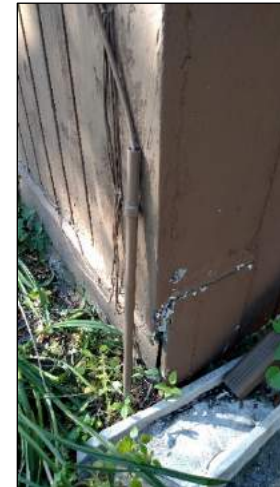
Fig. 8) Replaced wood piece plastered in with mortar-like substance. Note splash block. Photo taken facing southwest.
