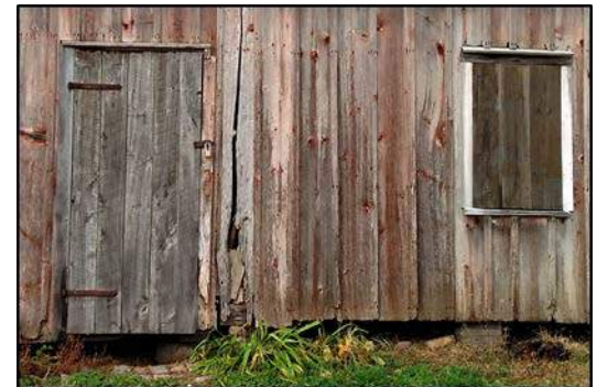
Fig. 14: Door hardware, decayed framing, broken wood and second boarded window space. Photo taken facing west.
