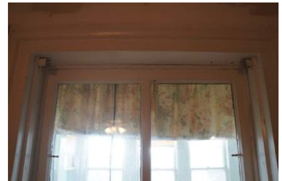
Window 6d- Missing Blinds
