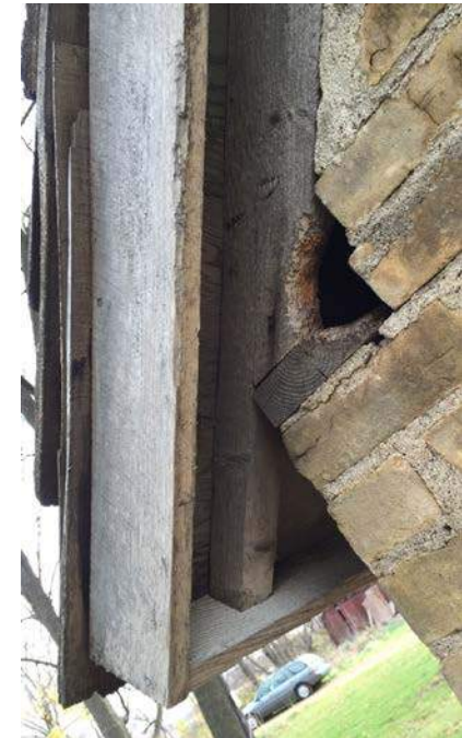
Figure 3: Damage to fascia on north elevation
