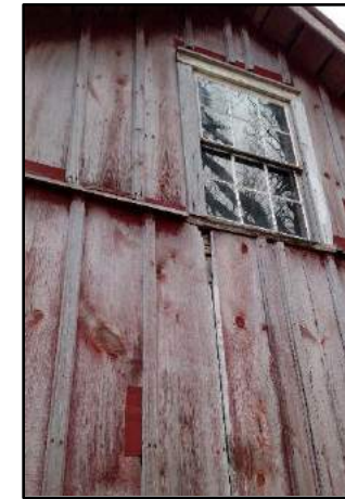
Fig. 5: Missing battens and metal patches. Photo taken facing southwest.
