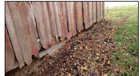
Fig. 6: Example of lower edge board and batten decay and wood-stacked pier. Photo taken facing southwest.
