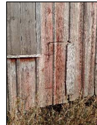
Fig. 12: Small hinged door nailed shut with worn board. Photo taken facing north.
