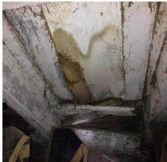
1.29 Floor damage seen from lower level
