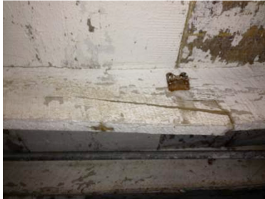
1.5 Joist cracking at mid-span
