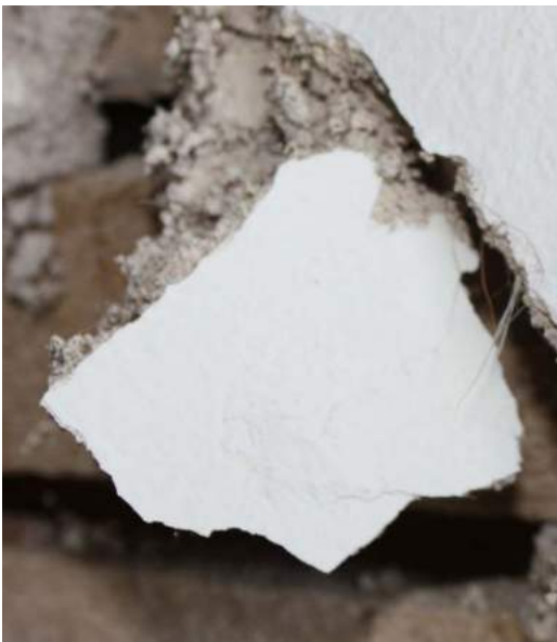
Figure 11. The horse hair matrix is clearly visible in this damaged portion of the wall.
