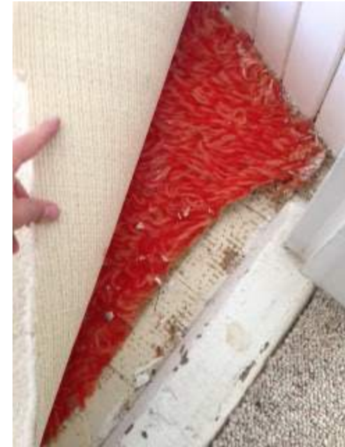
Figure 12. Two layers of carpet, thick adhesive, and paint layers of varying thickness cover much of the floor area.
