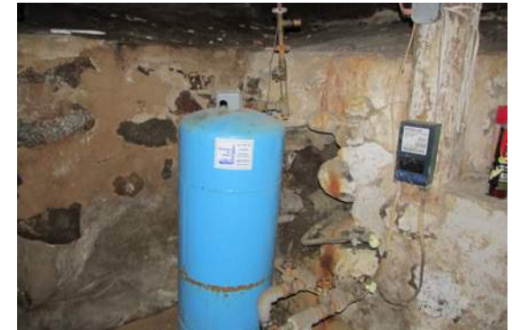
Original Basement- Water Well Pump
