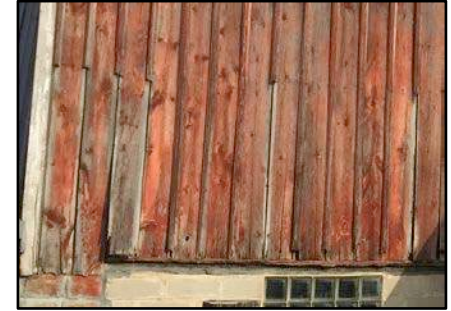
Figure 10: Missing parts of the wood battens.
