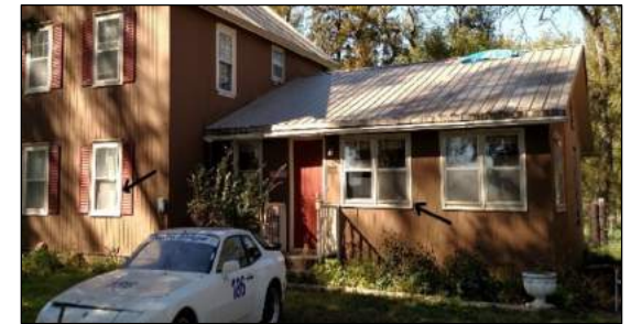
Fig. 10) Identification of windows with broken screens and storm windows. Photo taken facing south west.
