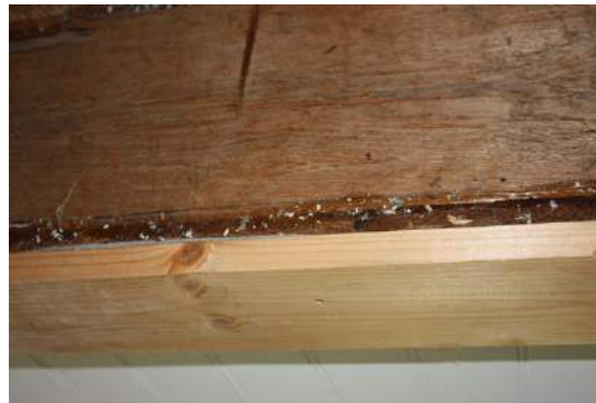
Figure 14. The ceiling structure is revealed at the opening to the attic. The plain board around the opening is not original to the building.
