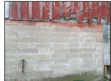
Figure 5: Efflorescence in the concrete block foundation, and deterioration of the wood.
