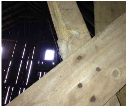
1.25 Close-up of Bracing Timbers with PPB Damage
