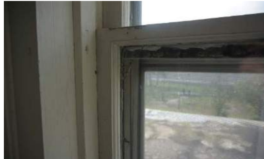
Figure 6. Window #5, lites (7) and (9) are damaged.
