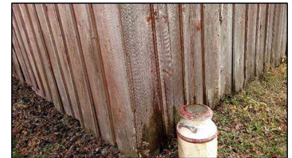
Fig. 10: Rising damp and moss. Photo taken facing
