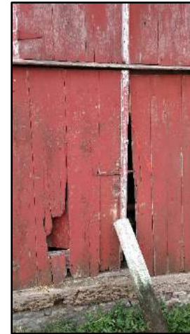
Fig. 7: Lower swing doors with breakage. Photo taken facing south.
