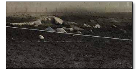
Figure 9: Stone foundation crumbling.
