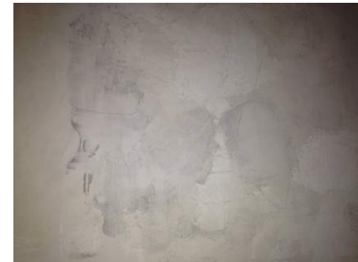
Room 2 Wall Damage
