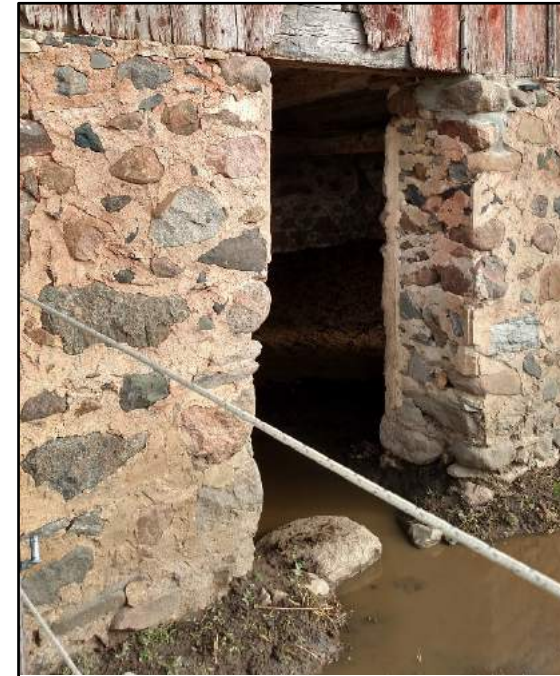
Fig. 15: Foundation opening, standing water, and surface grouting. Photo taken facing north
