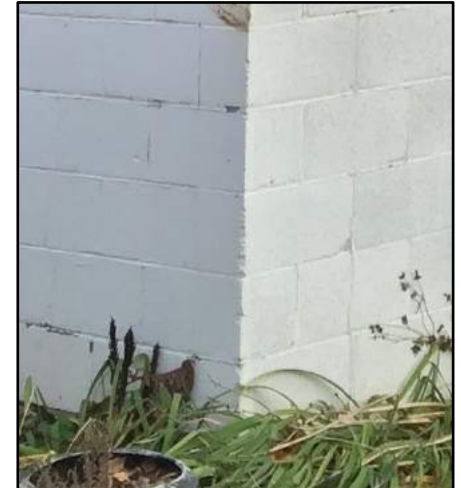
Figure 7: Concrete chipping at the corners.
