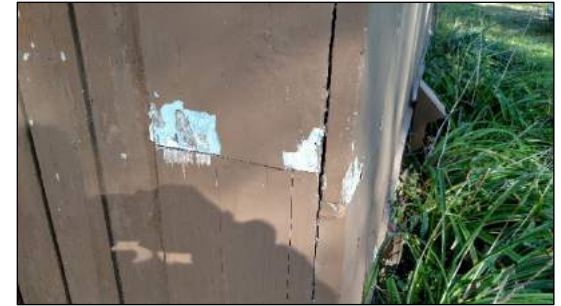
Fig. 7) Flaked off paint revealing white and then blue paint beneath. Photo taken facing north.
