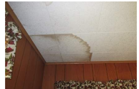
Room 4- Ceiling Water Damage in Southwest Corner
