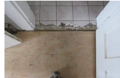
Room 7- Damaged Bathroom Tile
