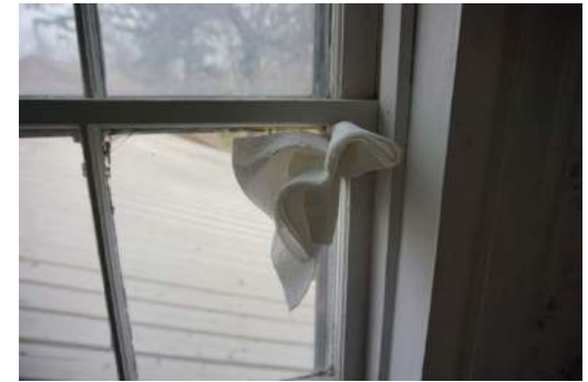
Figure 3. Window #2, lites (3), (9) and (12) are damaged.
