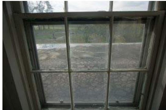
Figure 7. Window #6, lite (7) is damaged.
