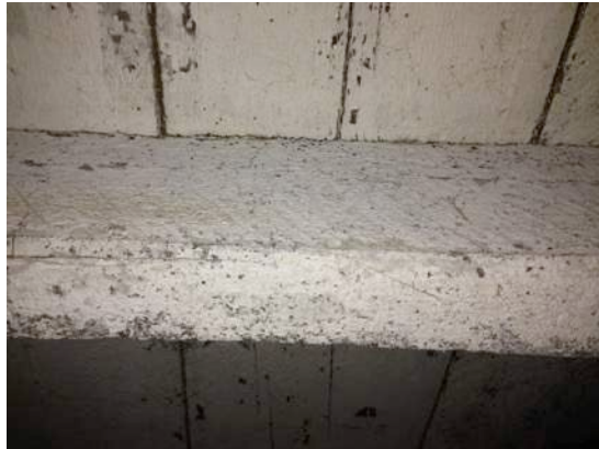
1.8 Close-up of joist condition. Evidence of PPB holes
