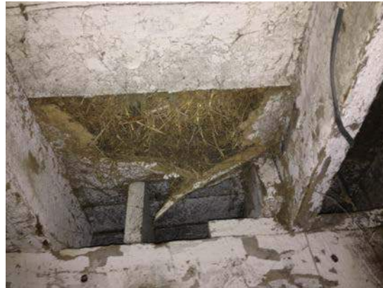
1.28 Floor damage seen from lower level
