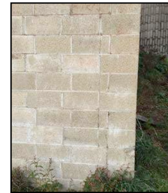
Figure 12: Concrete chipping at the corners.
