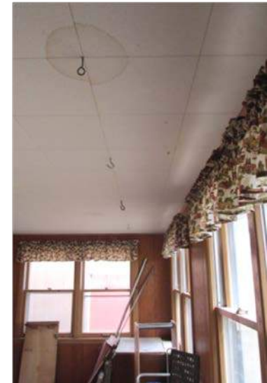
Room 4- Ceiling Water Damage
