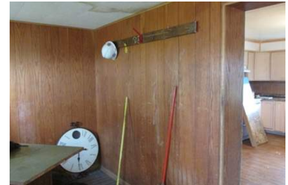
Room 4 Water Damage on West Wall
