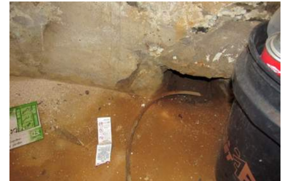
Basement- Hole in Foundation by Main Stairs
