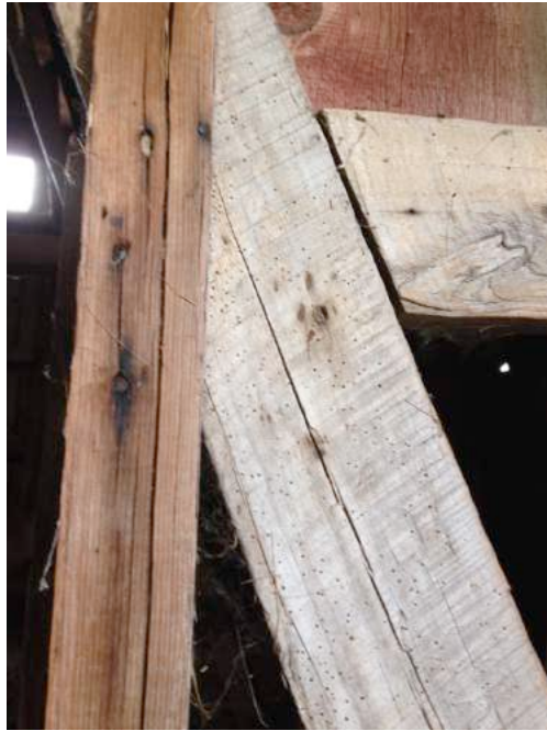
1.24 Close-up of Bracing Timbers with PPB Damage
