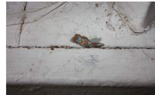
Figure 13. Poorly applied, thick layers of paint on the floor near the stair railing.
