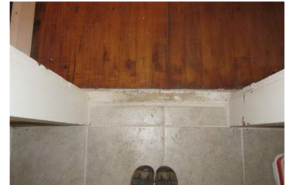
Room 1 and 3 Flooring Transition
