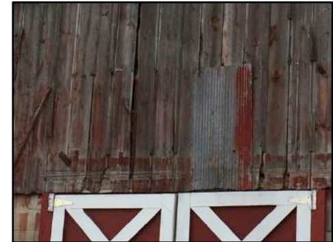
Figure 13: Metal sheet covering a missing part of the wood siding.
