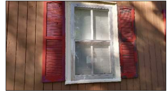
Fig. 9) Detail of window frame and shutters. Note condition and inappropriate addition of the aluminum storm windows. Photo taken facing west.
