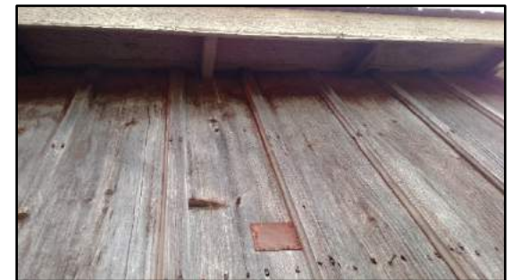
Fig. 8: One of many metal patches. Also shows condition of overhang and fascia. Photo taken facing west.
