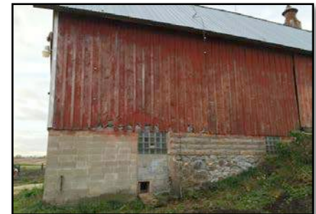
Figure 6: The triangular cut in the wood siding, and the discoloration of the concrete blocks.
