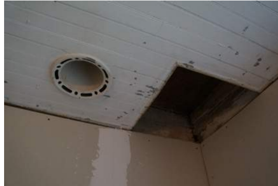
Room 5- Holes in Ceiling at Southwest Corner
