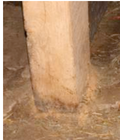
1.3 Evidence of PPB infestation – (above) Frass build up on around the column (right) Joist condition in lower level
