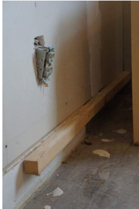
Room 5- Electrical Outlet with No Cover, Hanging Out of Wall, Missing Baseboard
