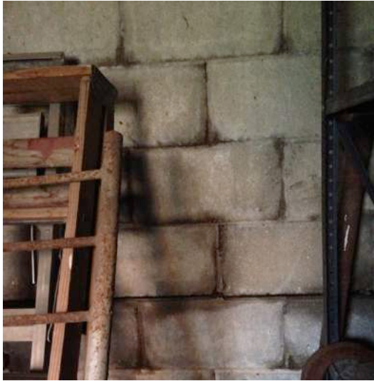
1.13 Mortar joints on East silo wall show evidence of water infiltration and a horizontal crack, above the first course in the photograph.
