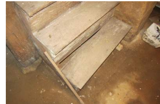
Basement Main Stairway- Broken Bottom Step
