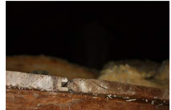
Figure 18. Old, dirty insulation should be removed.
