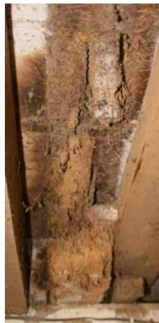
1.4 Joist failure from PPB. Interior damage of joist is visible.
