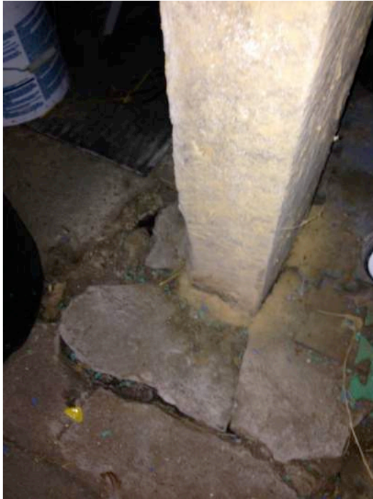
1.15 Evidence of footing failure
