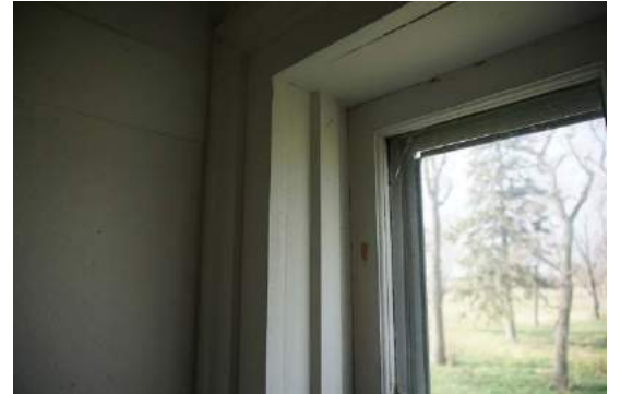
Figure 10. Window #9, lite (1) is cracked.
