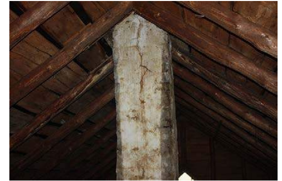
Figure 17. The chimney parging is cracked and discolored. Although water infiltration appears to have been halted, discoloration and insect nests remain.
