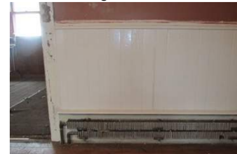
Room 3- Radiant Baseboard Heater
