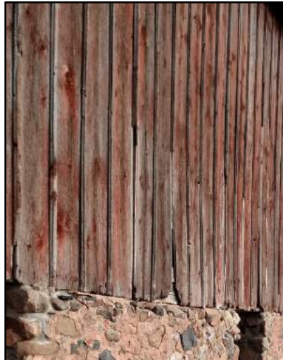
Fig. 13: Degraded boards, missing battens, and contact of boards on stone foundation. Photo taken facing northeast.
