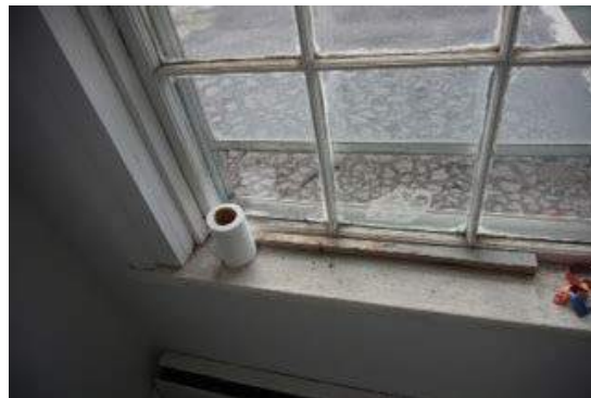
Figure 8. Window #7, lite (10) is damaged.
