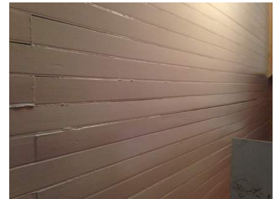
Room 3 Sagging Ceiling
