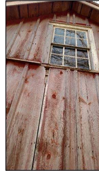
Fig. 9: Gable window, frame paint and weather wear, and exposed inner hand-hewn beam wall. Photo taken facing south.
