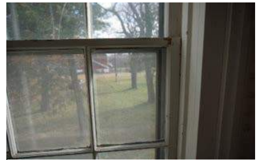
Figure 5. Window #4, lite (9) is cracked.
