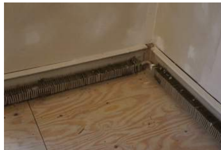
Room 6- Uncovered Radiant Baseboard Heaters on Southeast Corner
