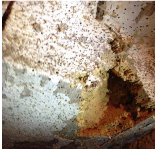
1.2 Evidence of PPB infestation - beam condition in Lower Level
