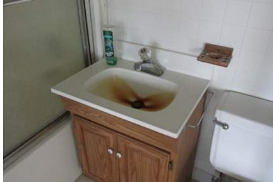
Room 7- Stained Bathroom Sink
