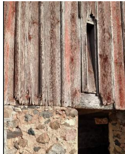
Fig. 14: Sill beam and broken boards. Photo taken facing north.
