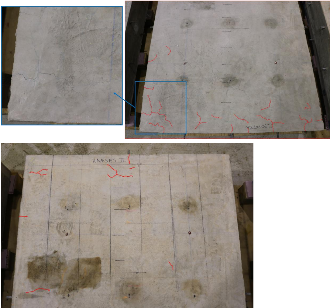
Figure 55. Visible cracking in south portion of slab 2 (top) and north portion of slab 1 (bottom).
