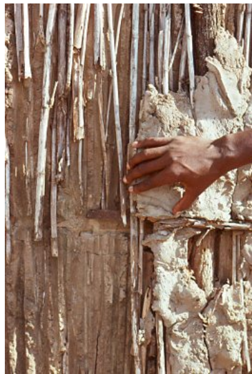
Fig. 3.6. A plastered wall, Maxaquene, mid-1970s. With time, plastered surfaces cracked, revealing the reeds within. (Source: Ingemar Sävfors)
