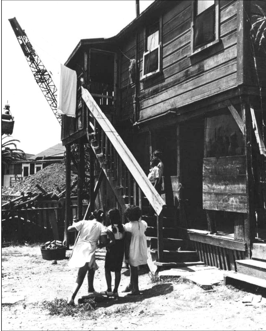
Figure 4.24. “Children watch Harbor Freeway construction,” 1948. As in other U.S. cities during the time, neighborhoods in Los Angeles were split in two as freeway construction followed the path of least political and economic resistance. Nadel captured this demolition scene in Downtown just before going to work for the LAHA. LAPL Photo Collection.
