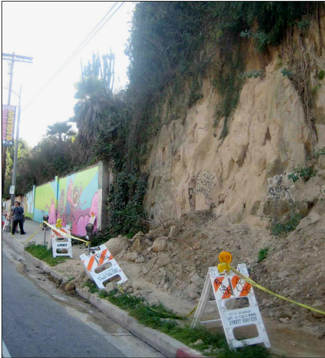
Figure 6.18. A landslide adjacent to one section of the Sunset retaining wall (a portion of Los Angeles: untitled is visible at left), 2011. Notice also the presence of graffiti tags on the exposed sandstone hillside. Photo by Stefano Bloch.
