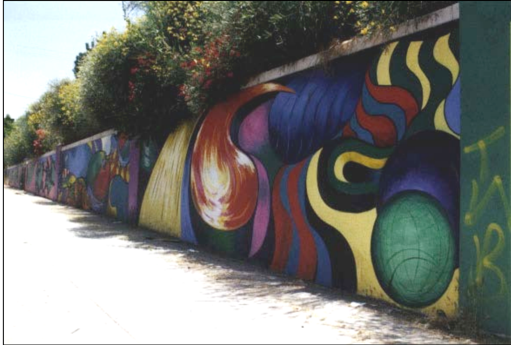
Figure 6.7. The western-most sections of the Sunset retaining walls as it appeared soon after De La Loza painted it in 1996.
