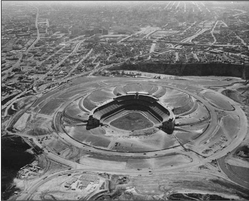
Figure 4.51. Looking east, Dodger Stadium and its expansive parking lot under construction, c.1961. L.A. City Clerk's Office.
