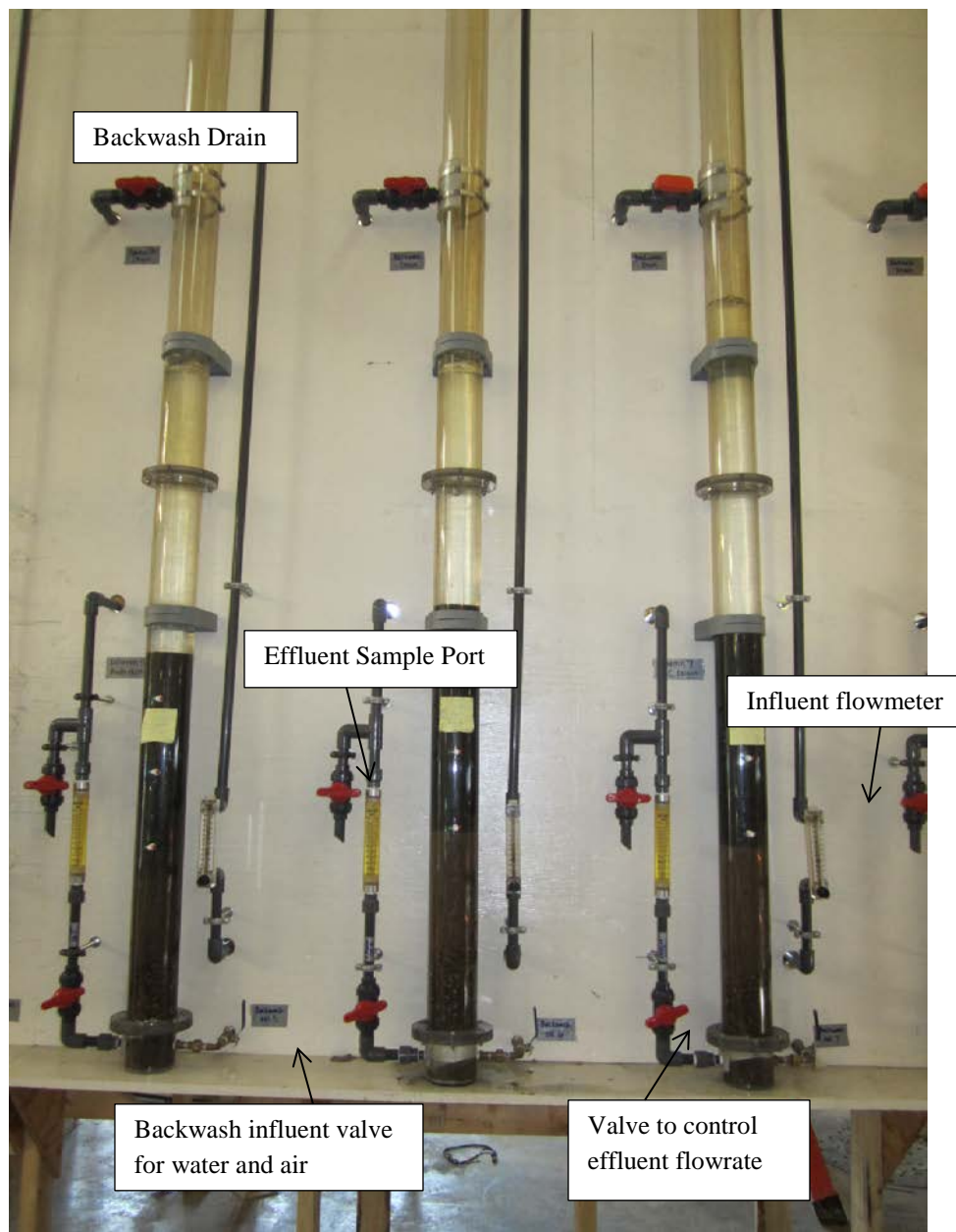
Figure D.7. Photo of three columns pointing out the valves and flow meters for the influent, effluent, backwash, and sampling port at MWTDS.
