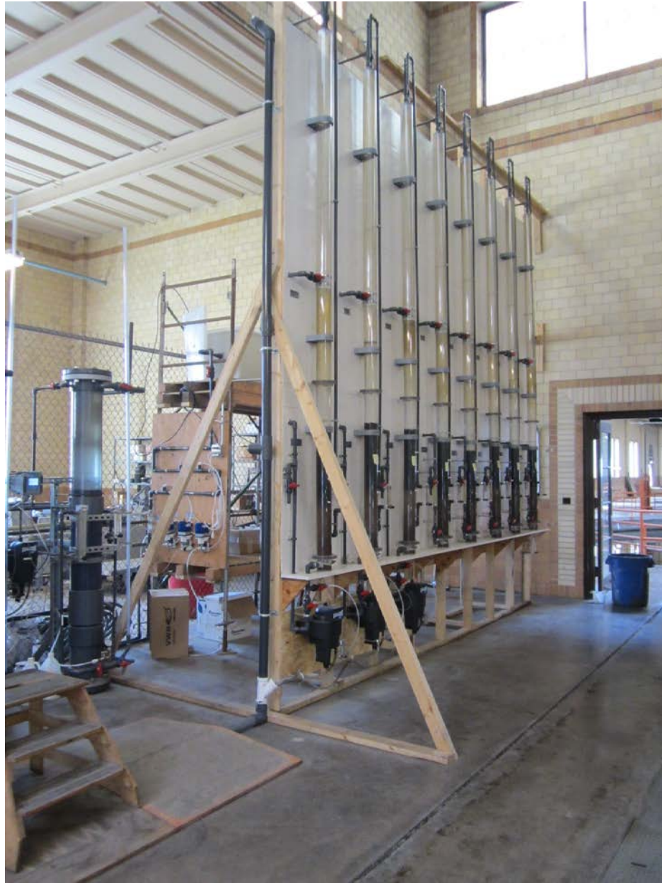
Figure 3-2. A photo of the pilot-scale column set-up at MWTDS for studying biologically active GAC.
