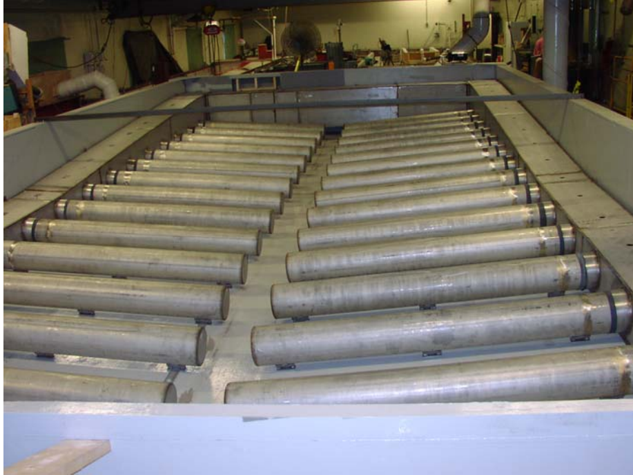
Figure 3. The basin with Johnson Screens underdrain system installed.
