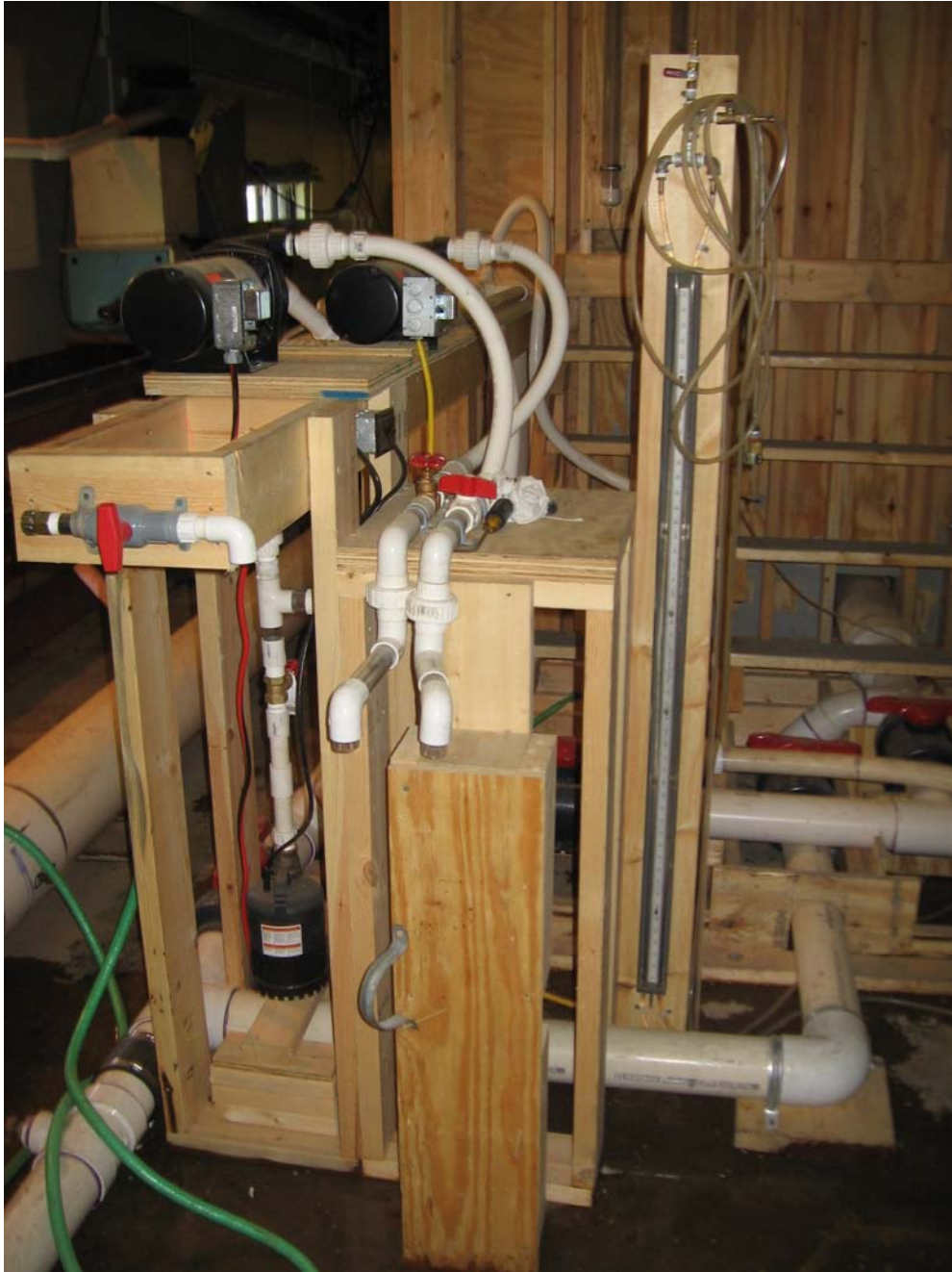
Figure 2.6. The pumps and plumbing used to measure the flow withdrawn from the flow chamber during the backwash mode.
