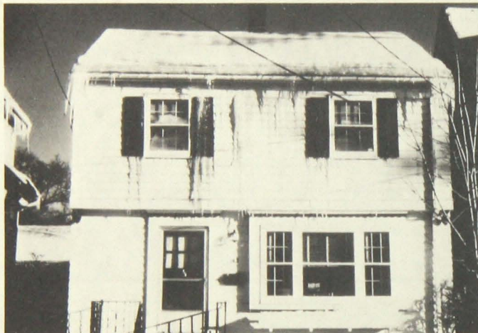
Figure 4. Frozen sidewall leaks emanating from ice-blocked eave.
