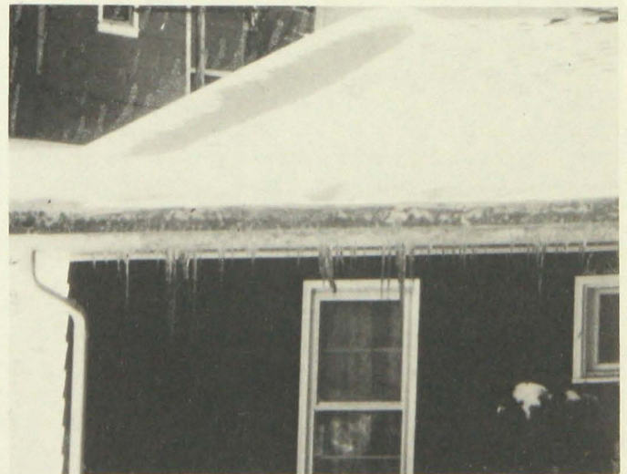
Figure 15. Telescopic lens photo of shrinking and sagging roof-snow on a modern (1962) roof.
