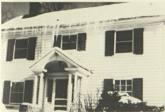
Figure 25. Well-insulated house built in 1933 with its almost annual eave-ice-dam.
