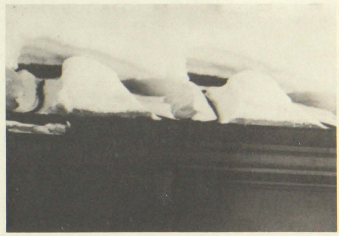
Figure 8. Secondary ice-dam developing uproof above heat zone of electric cable.
