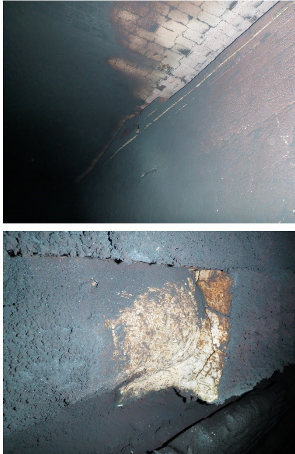
Figure 19: Furnace No. 6 Northshore Mining - Silver Bay, MN - 2012
