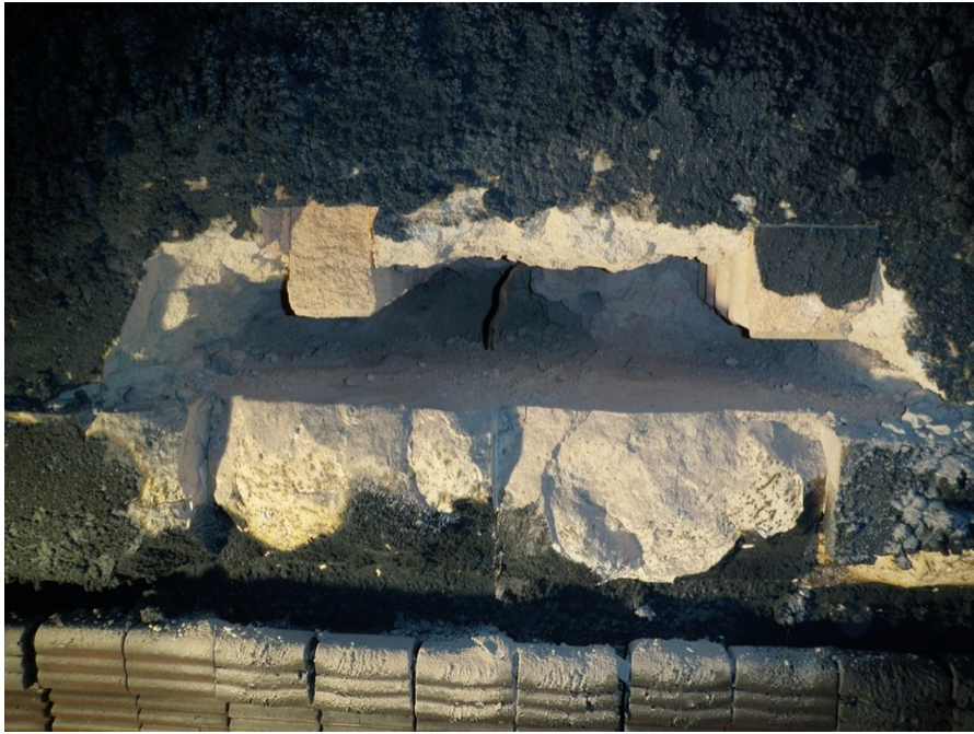
Figure 40: In-service Furnace 6 Curbs, before Extraction
