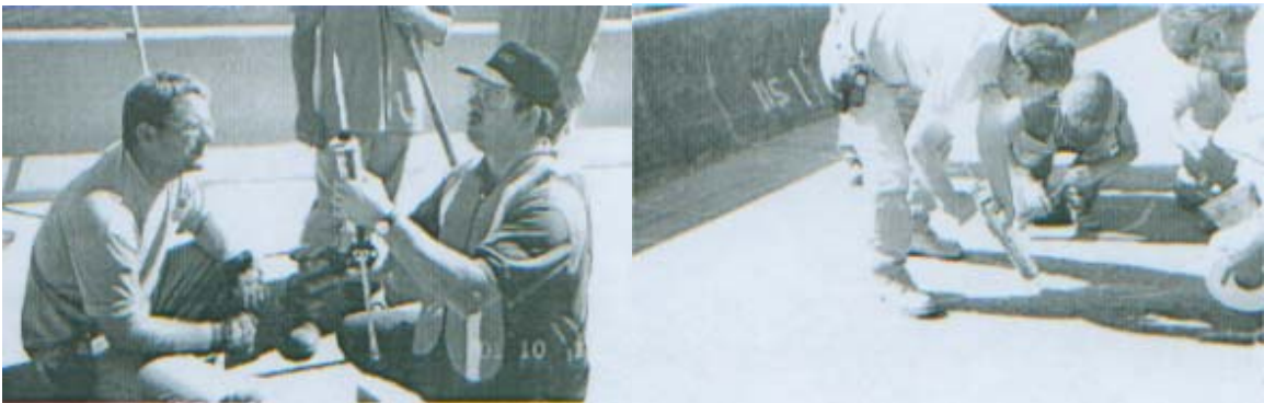
Figure 16 and 17: Examples of sealing individual cracks (Soriano 2002)
