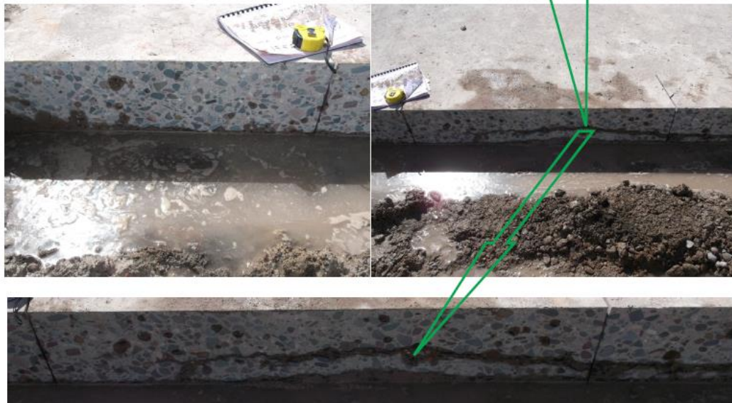
Figure 5-33. SAFT Panoramic reconstruction and comparison with the actual delamination crack path at 18 in. from Joint #2 in the approach slab.
