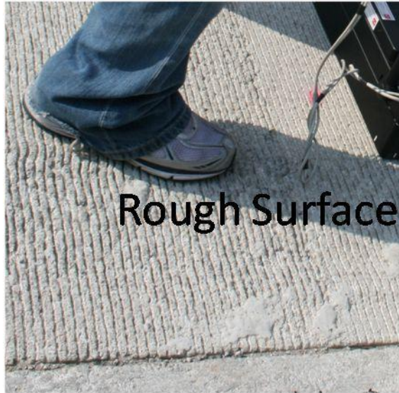
Figure 5-5. Example of a rough surface that required the device to be move to the left for proper coupling of the transducers.
