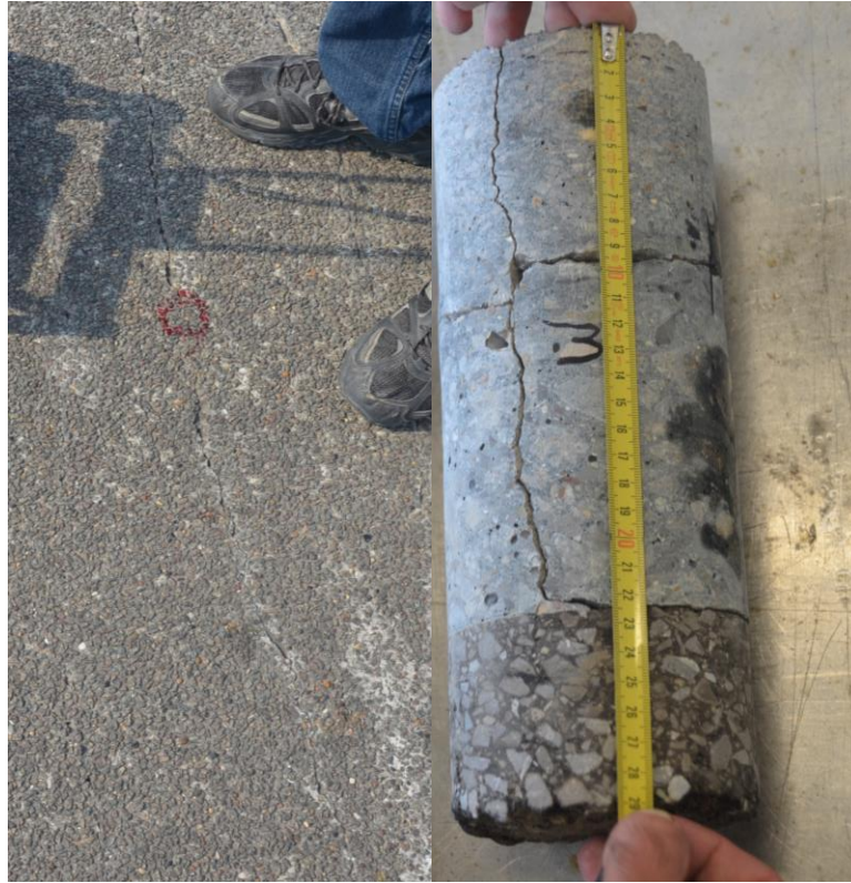
Figure 4-10. Forensic verification of the delaminated concrete condition with vertical crack.
