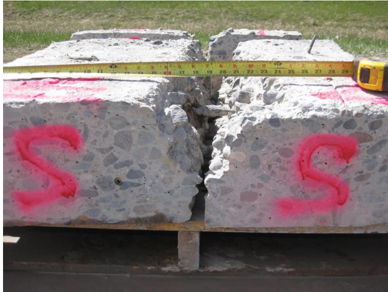
Figure 5-30. Example “tenting” distress observed at joint 2, in both approach and leave slab #2 as viewed from the south side of the slab.
