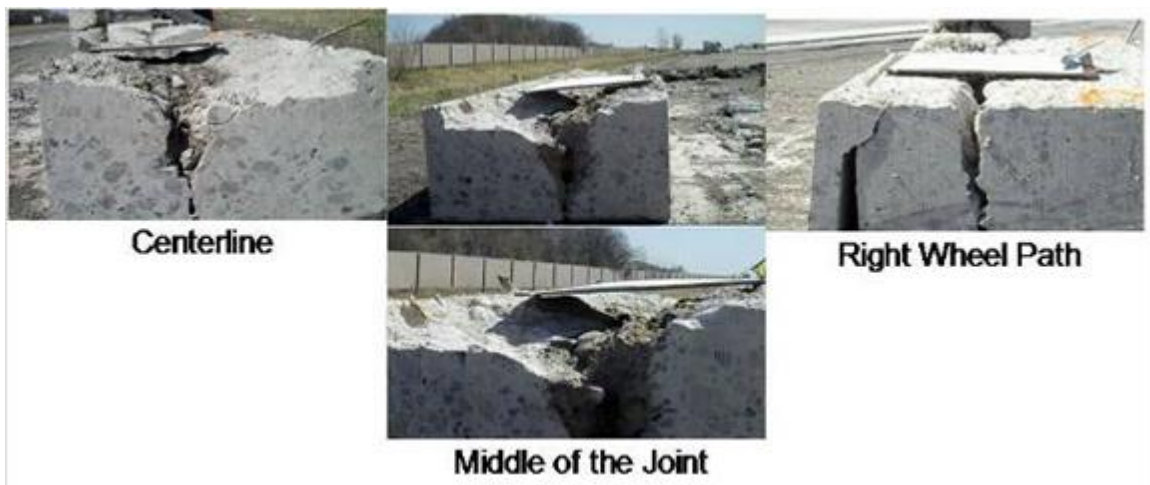
Figure 5-25. Forensic sample sections used to verify the concrete condition on the underside at various locations near the transverse joint.
