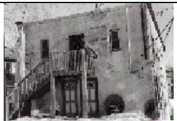
Photo D: a water damaged apartment building
