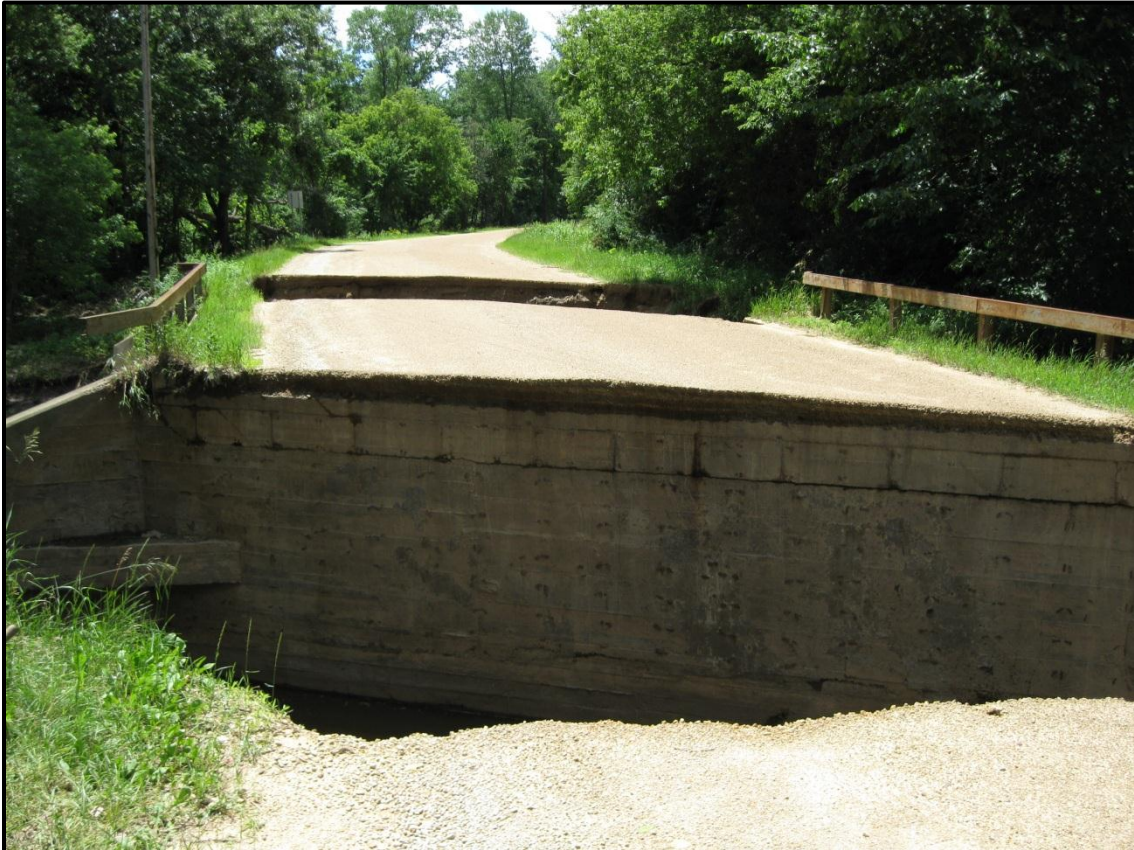
Figure 24: Picture of Bridge on the East Branch of Trout Brook: X1. (Location of X1 is shown on Figure 2.) This wash out damage occurred from the 14-15 June 2012 flood.
