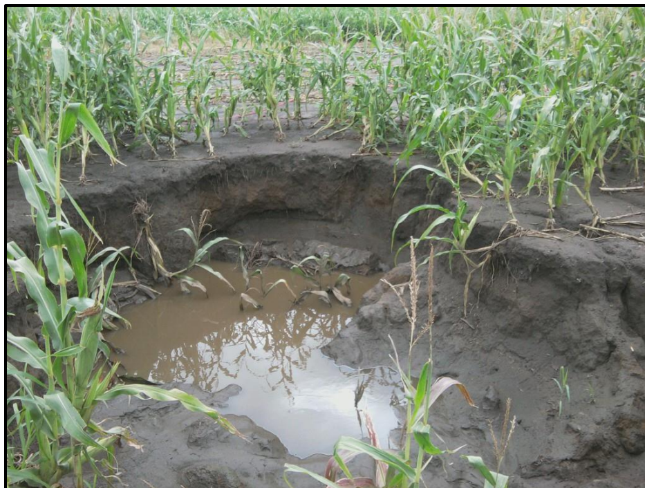
Figure 23: Picture of Sinkhole D11. (Location of Sinkhole D11 is shown on Figure 21.) This sinkhole formed due to the 14-15 June 2012 flood and was discovered afterwards. Picture is looking east.
