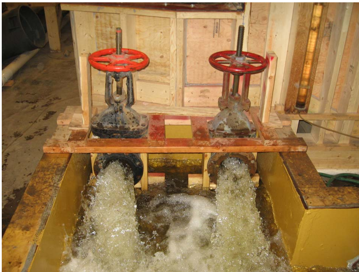
Figure 7. The 6-inch gate valves on the draft tubes.
