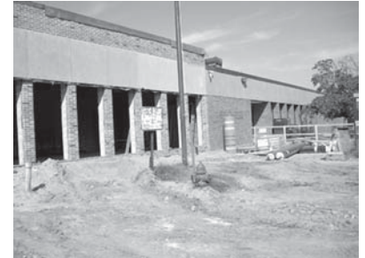
Old meets new at the Cereal Disease Lab. New construction almost doubles research and office space.
