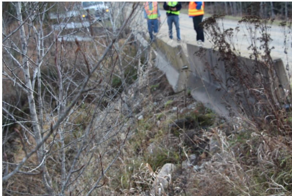
Figure 36: St. Louis County slope and displaced concrete barriers
