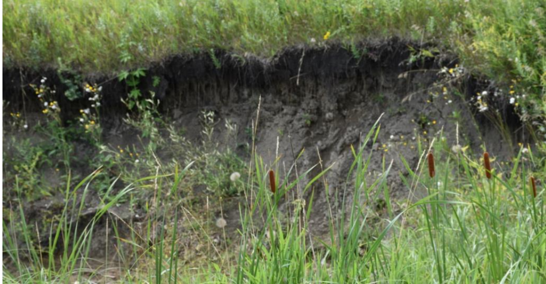
Figure 33: Pennington County site slope, clear rotational failure
