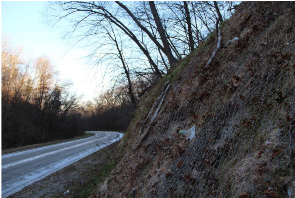
Figure 39: Wire mesh and rock bolt cover at Washington Co. site
