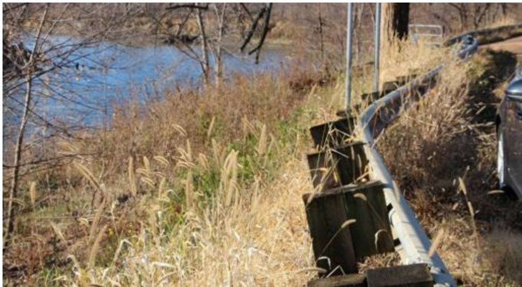
Figure 20: Carver County site slope, crooked guardrails indicate soil creep
