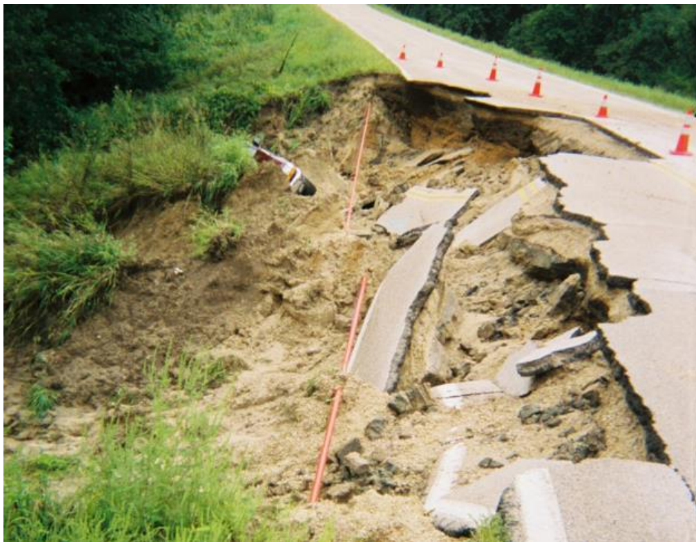
Figure 1: Example of damage from slope failure (from Houston Co. Highway Department)
