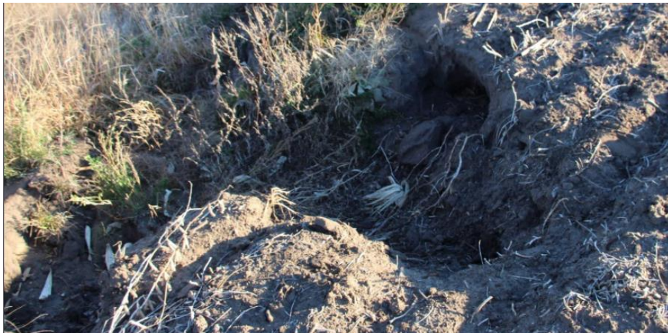
Figure 28: Erosion at edge of planted field causes slope failure at the Lac Qui Parle Co. site
