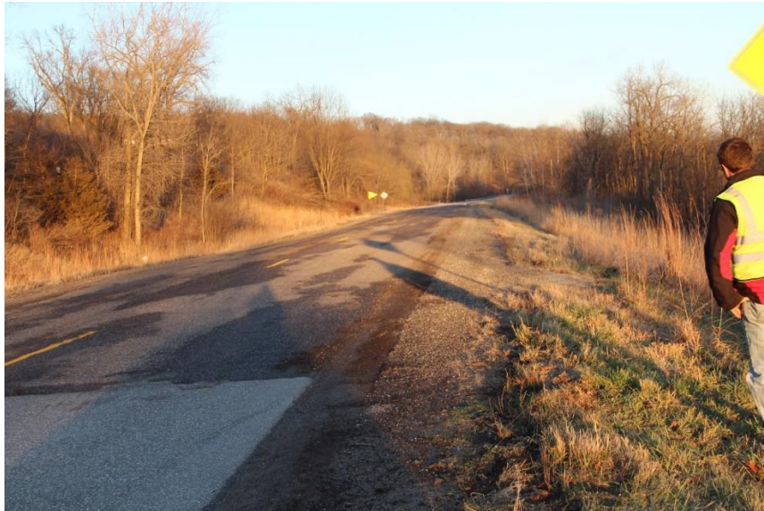
Figure 21: Pavement distress at Fillmore County Site
