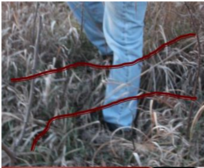
Figure 23: Scarp face at edge of failure at Fillmore County site
