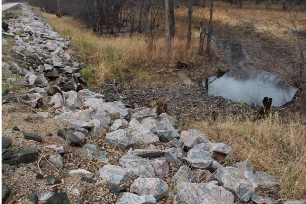
Figure 34: Failed (east) side of Redwood County site slope and nearby stream
